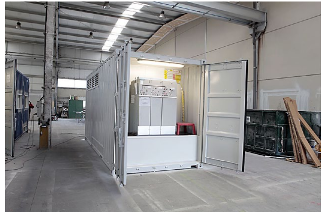
GP Tech's APIS indoor covering tests for the cULus certification
